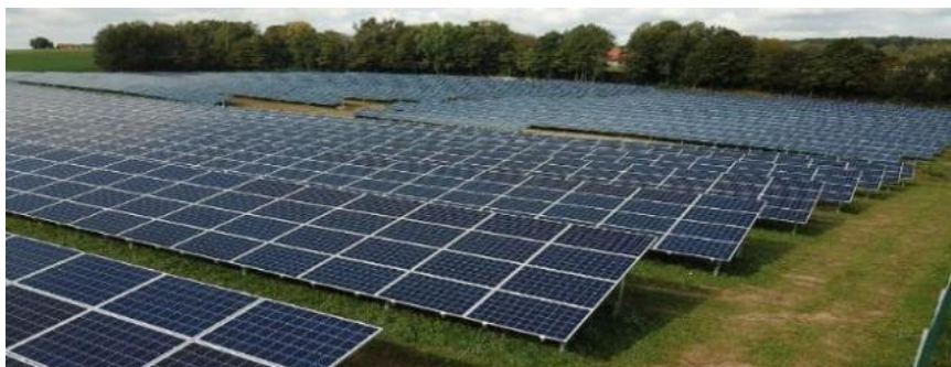
Figure 17. Solar PV park.
